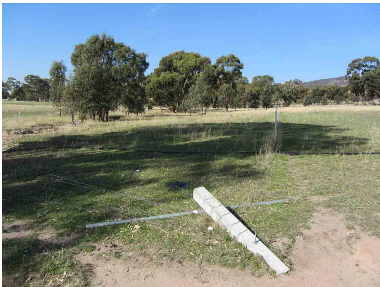
Figure 1.1 – Concrete end assembly damaged by 2012 flood, tributary of the Six Mile Creek, Baringhup, north-central Victoria (photo: North Central CMA)
