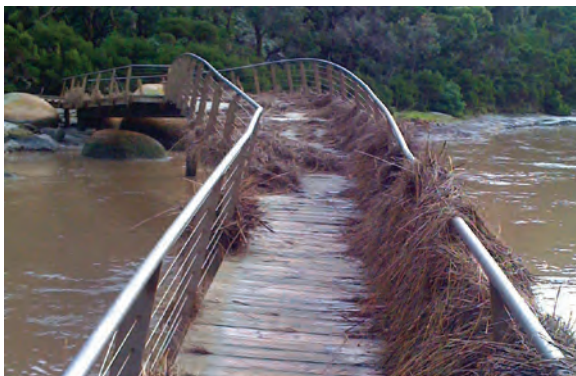
Flood debris, Tidal River, Parks Victoria
