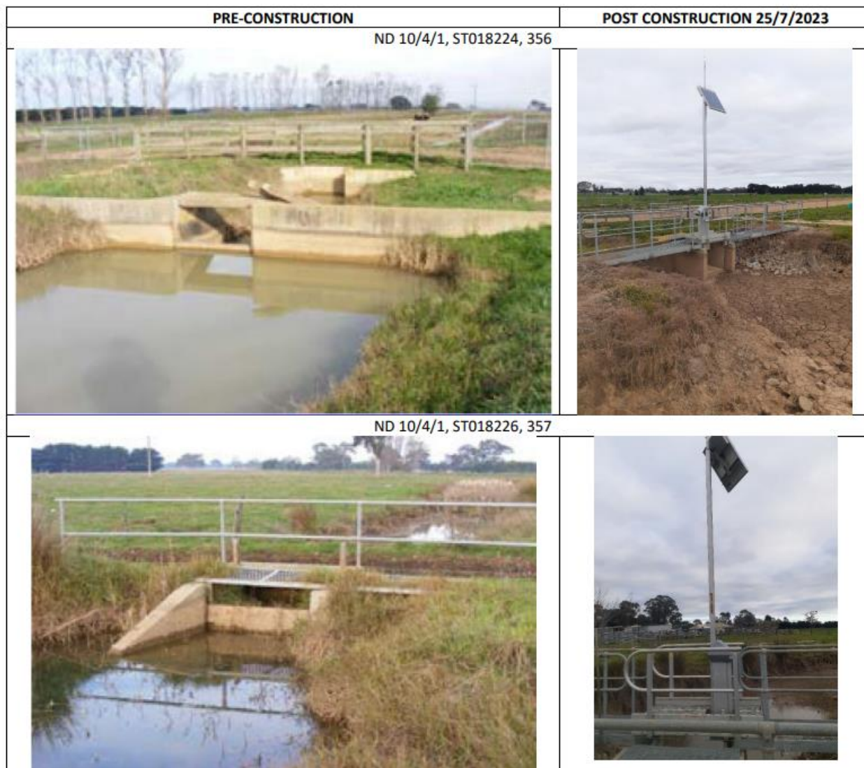
Figure 5-1 Photos of ST018224 and ST018226 before and after upgrade
