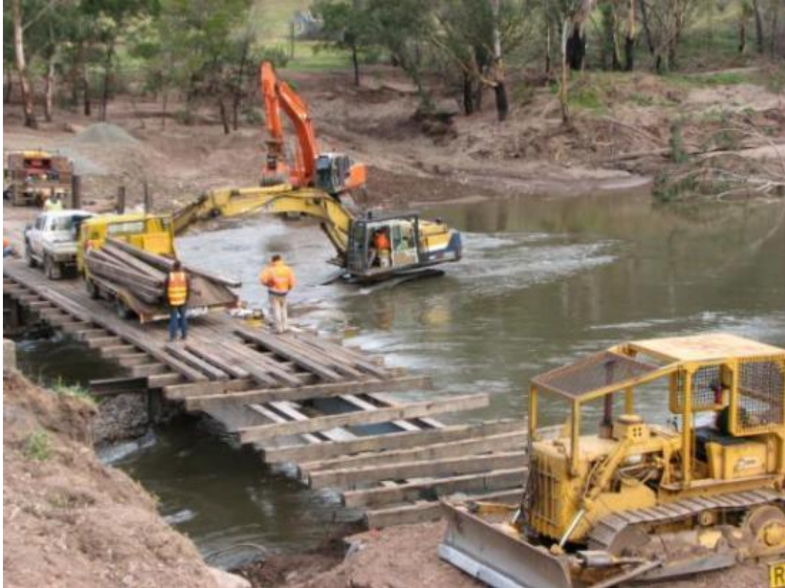
Figure 4. Temporary bridge construction over Macalister River following loss of Cheynes Bridge in the 2007 flood event.
