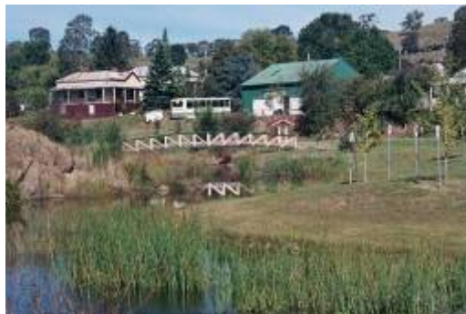
Livingstone Creek Omeo. Channel reconstructed following 1999 flood event to protect sewer main
