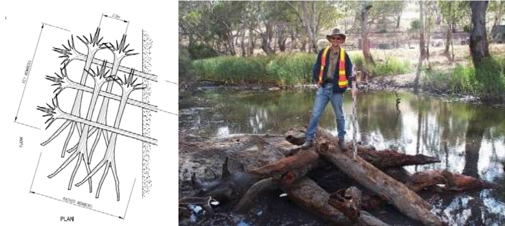
Engineered log structure schematic sketch (left) and in Glenelg River at Harrow (right) (Images courtesy of Earth Tech)
