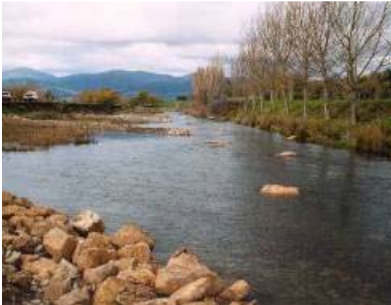
Bed seeding (right) combined with rock groynes for alignment training, Snobs Creek (Photo courtesy Paul Brown, Department of Primary Industries, Victoria)
