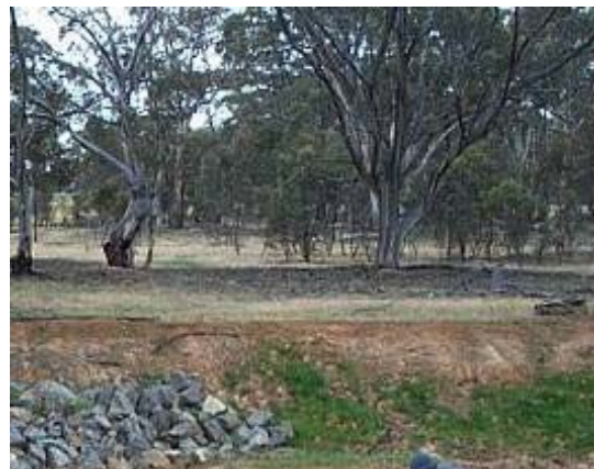
Battering combined with rock beaching, Wattle Creek, tributary of Wimmera River, western Victoria
