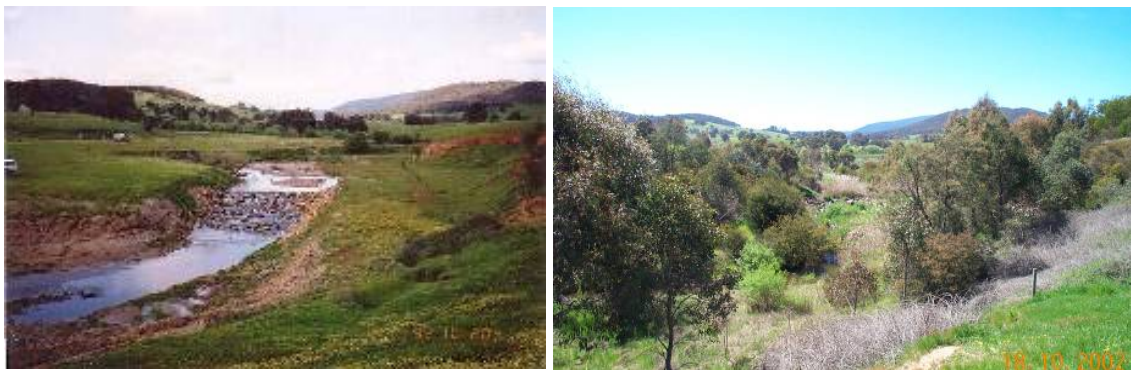
Figure 5.15 Barwidgee Creek, north east Victoria, six months (left) and 10 years (right) after rock chute construction and revegetation (Images courtesy of T. McCormack, North East CMA)
