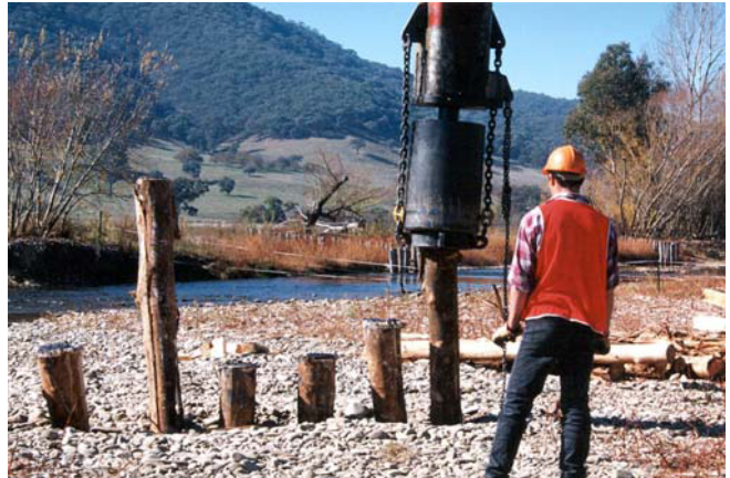
Timber piles in north east Victoria (Photo courtesy of North East CMA)
