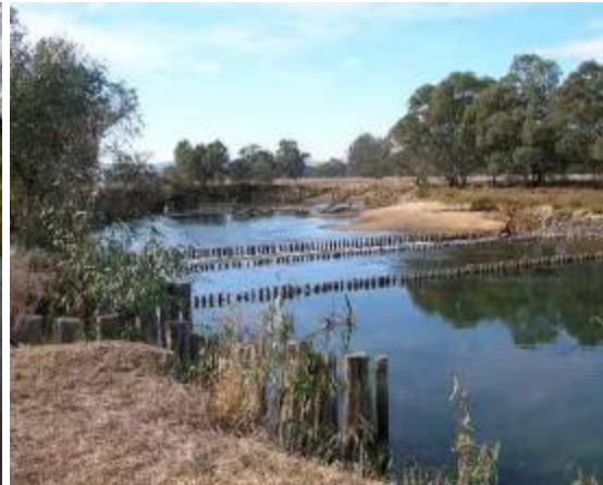
Avulsion management works including pile field and bed seeding Dights Creek, anabranch of the River Murray, NSW
