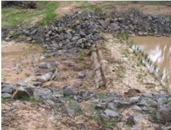
Log sill, with accompanying rock beaching, Wattle Ck, tributary of the Wimmera River
