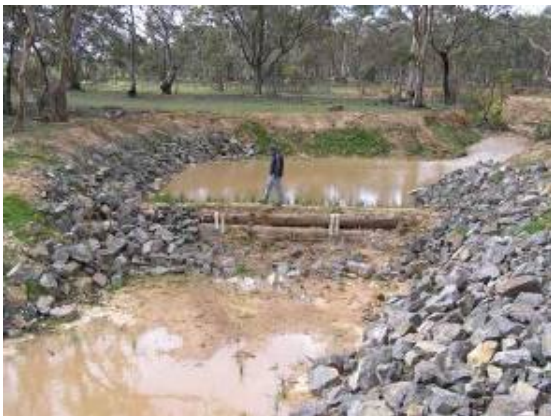
Log sill and rock beaching at Wattle Creek, Wimmera River catchment (Image courtesy of Earth Tech)
