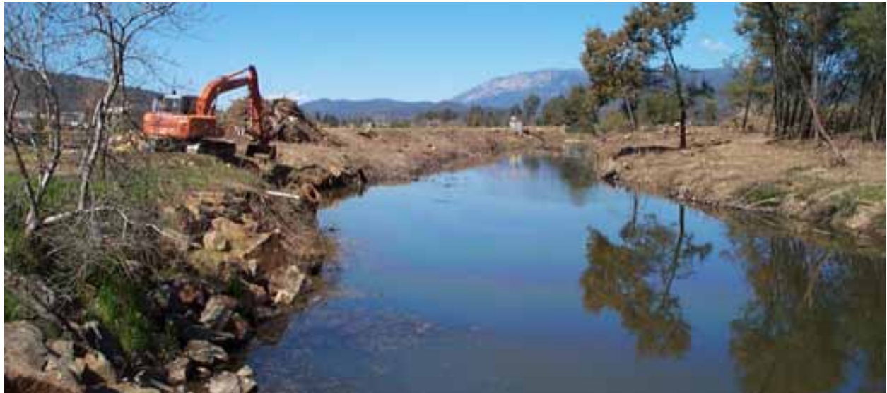
Willow removal on the Happy Valley Creek, Myrtleford. Photograph: North East CMA
