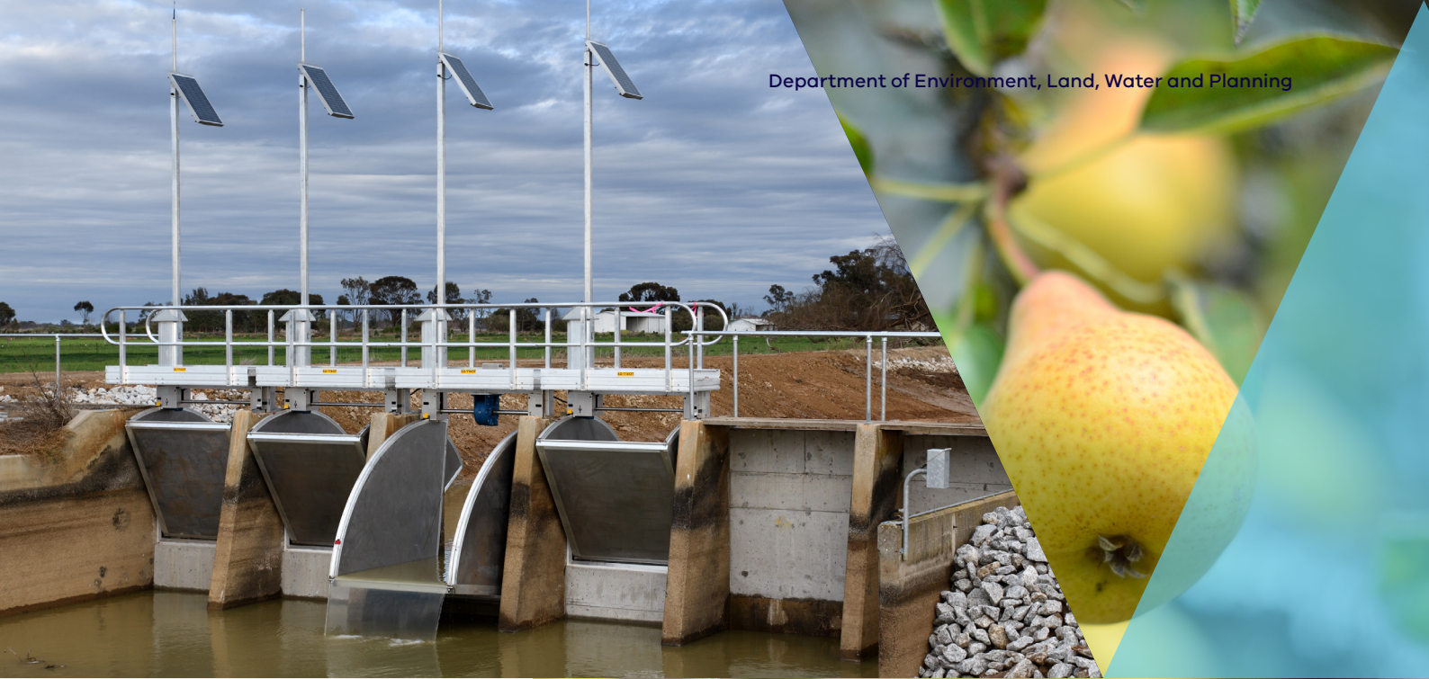
Modernised irrigation structure that measures and regulates flows in channel system. Courtesy GMW Connections.
