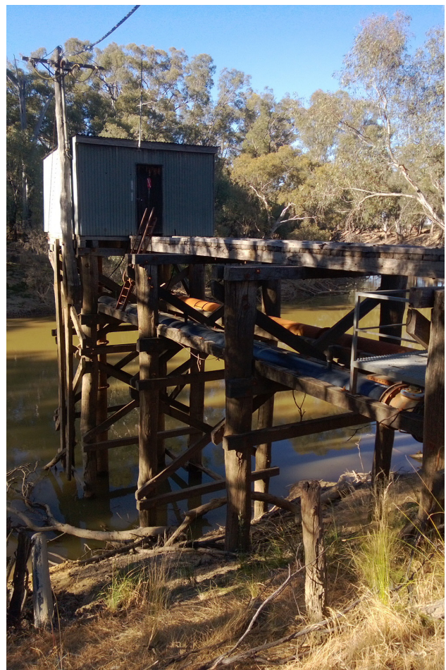
Wakiti Pump Station
