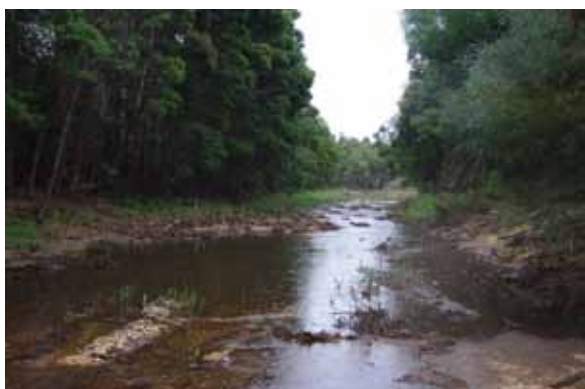
Removal of in-stream exotic vegetation (before and after photographs) in Creswick Creek at Clunes. Photographs: North Central CMA
