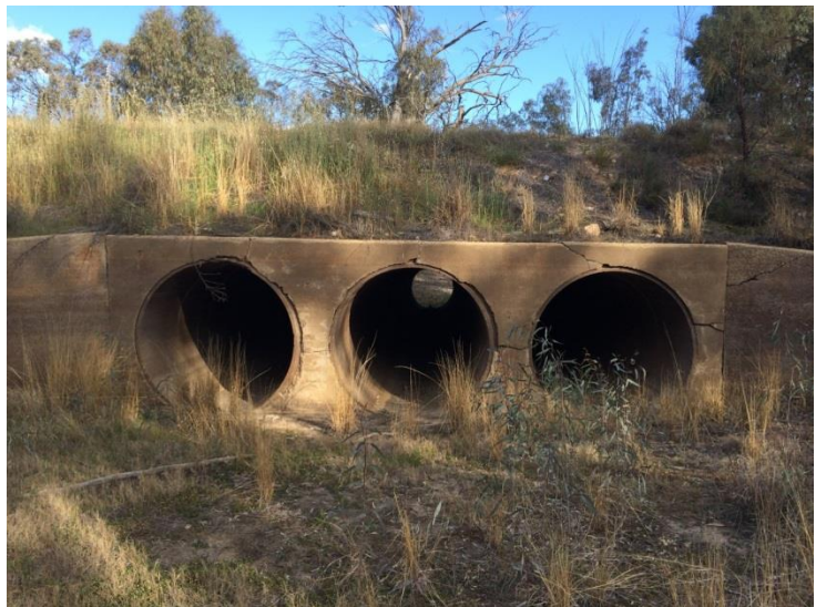
Figure 8. Culvert under Murray Valley Highway (from northern side of Highway, looking south)
