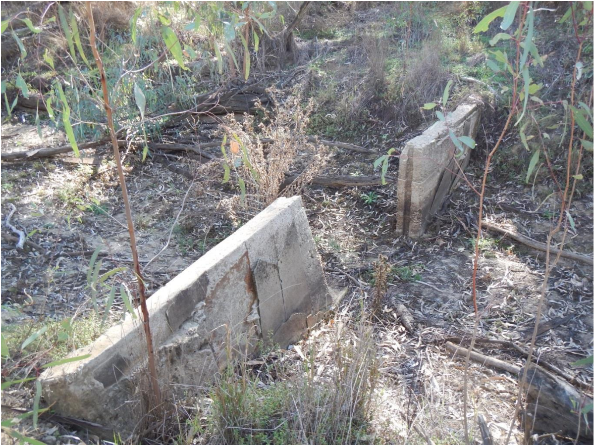
Figure 20. Photograph taken of a regulator structure in disrepair, this structure is located on the creek inlet to Central Fishers Lagoon.
