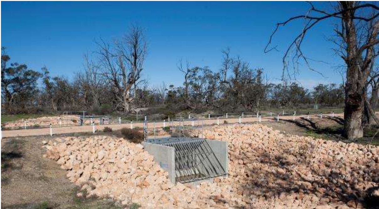
The Lake Wallawalla environmental regulator, constructed under The Living Murray program in 2006
