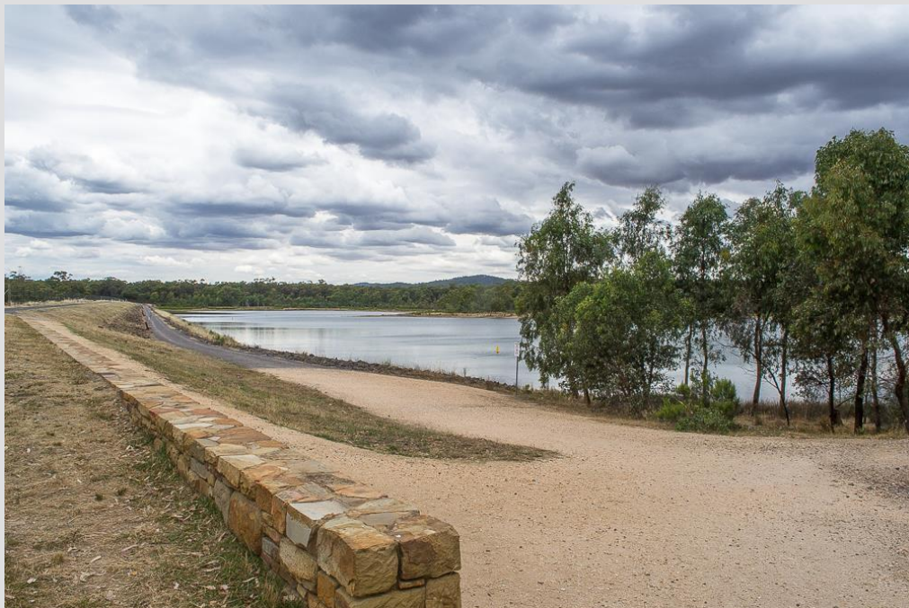
Figure 3: Crusoe Reservoir dam wall viewed from left abutment post partial decommissioning and showing reduced water level (Goldfields Guide, 2021)
