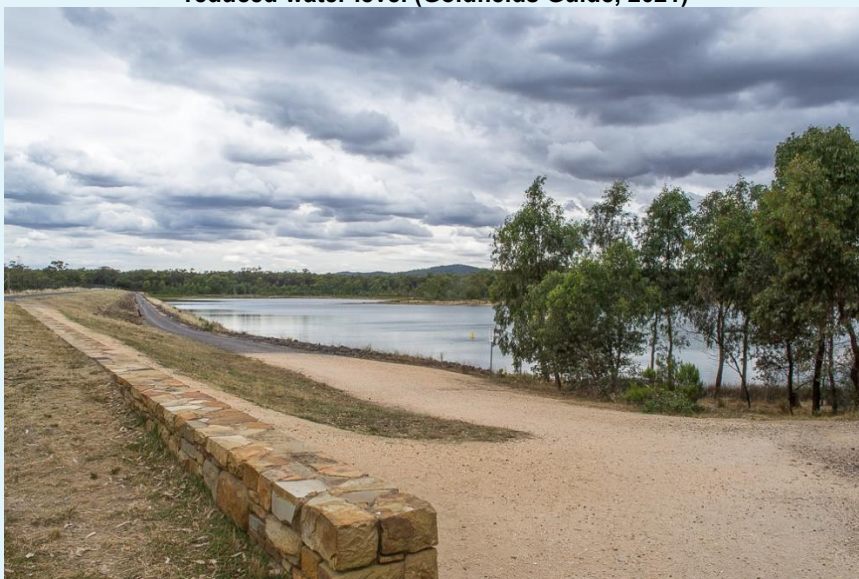
Figure 5: Crusoe Reservoir dam wall viewed from left abutment post partial decommissioning and showing reduced water level (Goldfields Guide, 2021)
