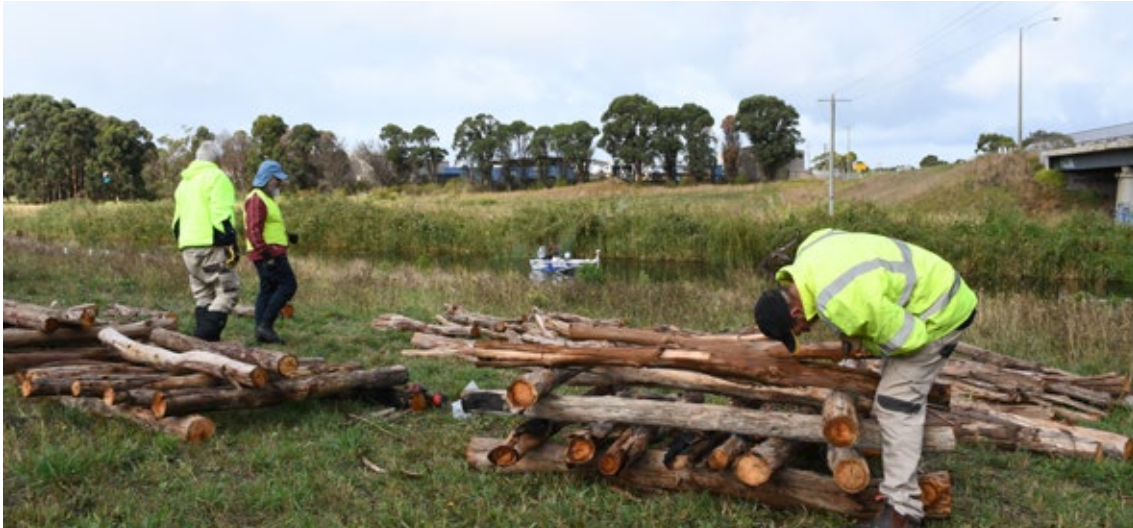
Figure 7: Volunteers constructing fish hotels on the banks of the Merri River in Warrnambool. Image courtesy of Glenelg Hopkins CMA.
