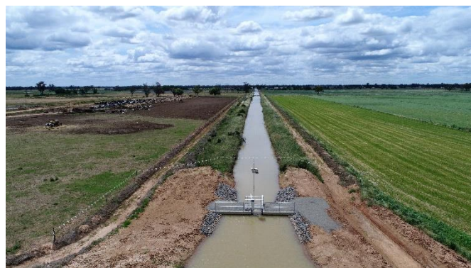
Figure 1: The Connections Project has modernised irrigation delivery infrastructure to reduce water losses, with works completed in all six irrigation areas of the GMID.
