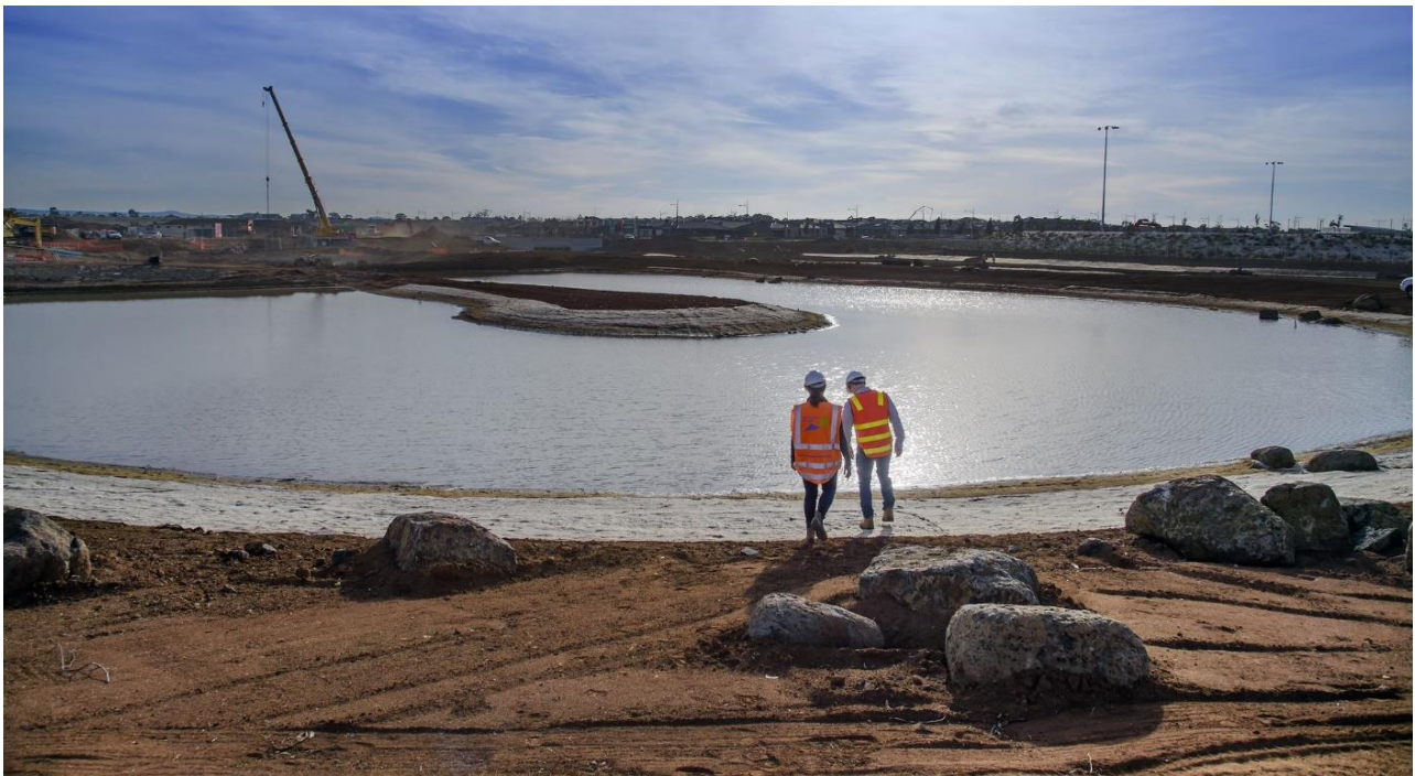
Toolern Stormwater Harvesting Project, Western Water Source: DELWP
