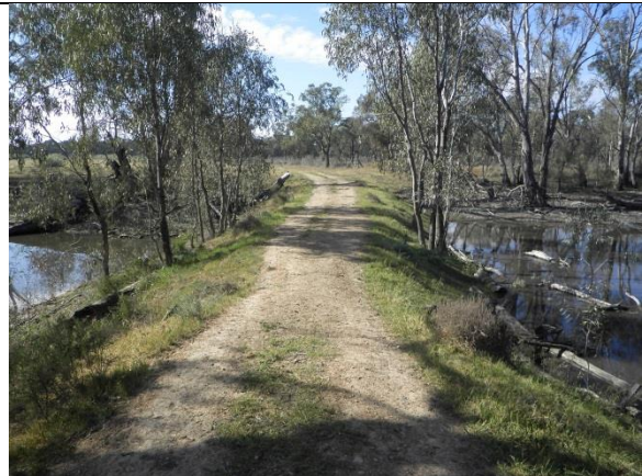
The private access track at Impediment 16. Note the difference in water levels from upstream (right) to downstream via the culvert (left).
