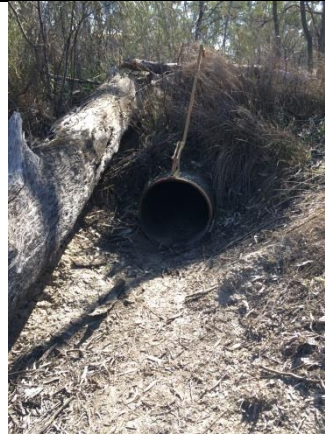
The upstream end of the pipe culvert at the cutting at Impediment 5. Evidence exists of past ability to close off the culvert.
