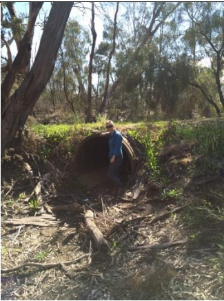
At Impediment 7, the road parallel to the channel and pipeline crosses the creek, with a large culvert enabling passage of creek water.
