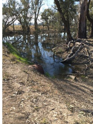
Impediment 19 (left of image) is an access track used by a private landholder. Pipe culvert and altered creek course is shown in the foreground.
