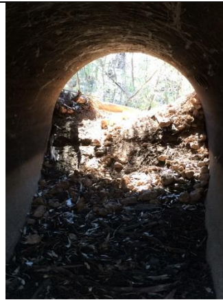
The downstream end of the culvert at Impediment 7, however, is partially blocked by soil and rubble.
