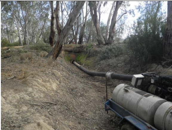
Pump Site C, showing temporary pump in foreground and pipe through Impediment 22. This is also River Connection Point C, looking away from river.
