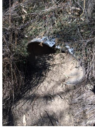
The ~600 mm diameter pipe culvert at the cutting at Impediment 5. This view is the downstream end.
