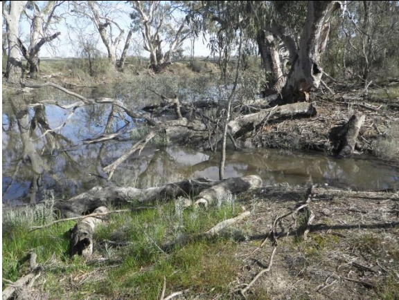
The downstream cutting exit to the creek at Impediment 17. Note the fallen timber at this point, which, if allowed to accumulate would further impede flow.
