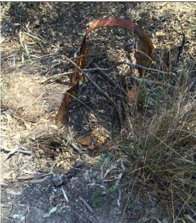
The aged pipe culvert at Impediment 6 is in worrying need of attention.
