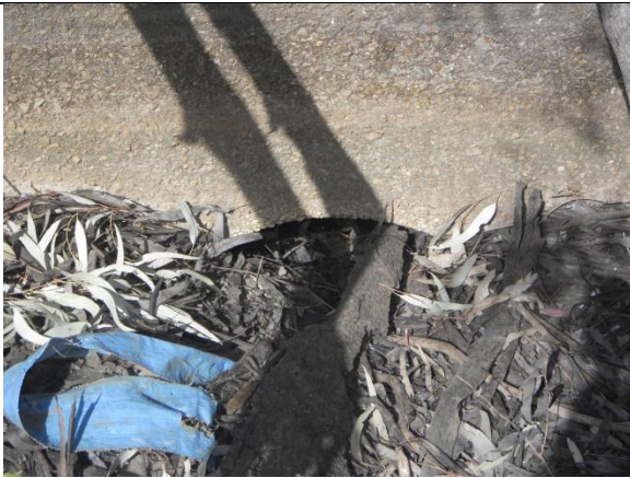
The downstream side of the pipe culvert at Impediment 9 under the channel. The culvert is of comparatively good size (~900 mm diameter), however a large volume of debris almost completely blocks flow.
