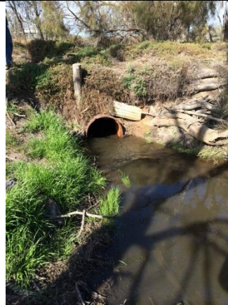
The culvert at Impediment 18, again diverting the creek flow to just outside the natural bank. Fast-flowing water can be seen entering the pipe, and evidence of logs removed from the entrance on right of picture.
