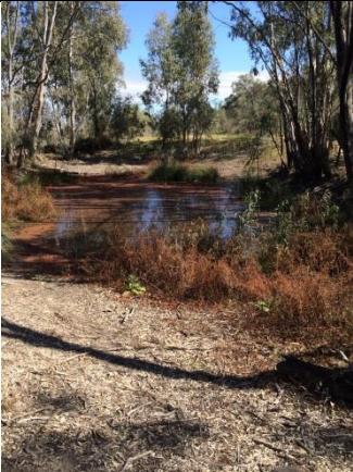
At Impediment 7, the irrigation channel enters a pipe and flows under the creek bed, reemerging once more into open channel. There is evidence of a leak in this wetland shown.
