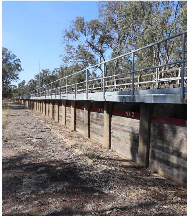
Figure 6: Regulator used as part of the Loch Garry Flood Protection Scheme
