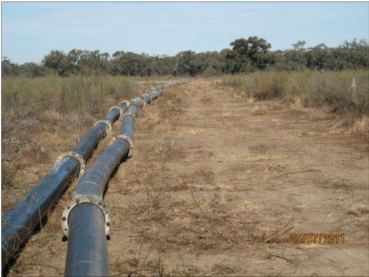
Temporary pipes used to delivery environmental water to Lakes Powell and Carpul (2011)
