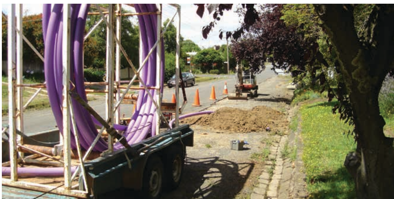
Coliban Water purple piping
