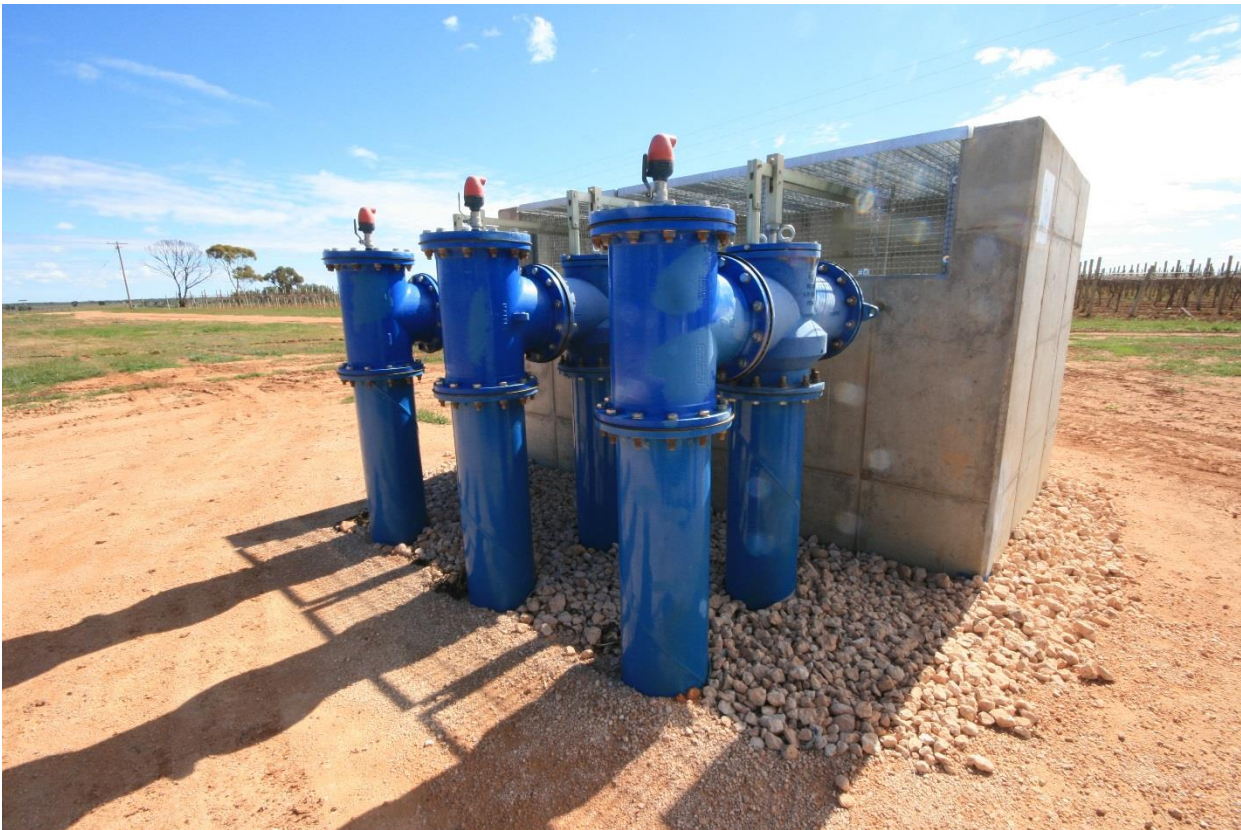
Water delivery infrastructure is being modernised in Sunraysia, including underground piping with structures like these pipes that manage water pressure.
