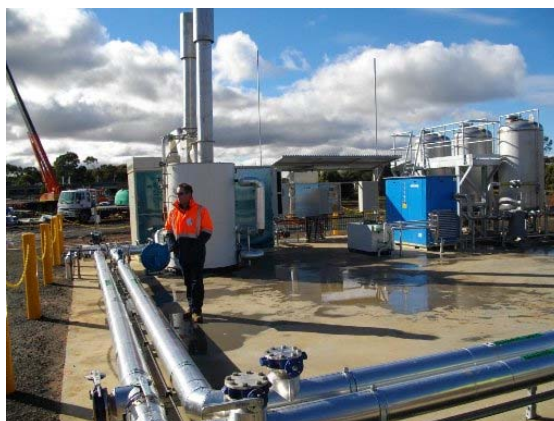
Above: The cogeneration plant at Western Water's wastewater treatment plant, Melton South, takes excess heat from the burning of methane and uses it to heat water which circulates in a sleeve round the sewage sludge. Digestion is accelerated and more methane is produced.
