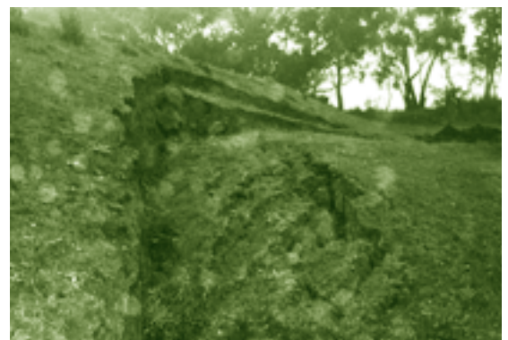
Embankment slip due to poor construction
